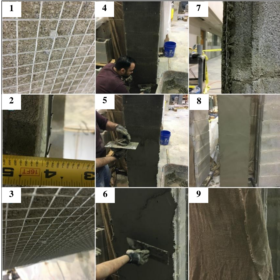
Figure 6.2 WWSM plastering process, (1) securing WWSM using hot-glue silicon at selected spots, (2) checking spacing between mesh and substrate, (3) masonry spraying with water, (4-6) applying mortar overlay, (7) checking overlay thickness, (8) overlay surface troweling, and (9) curing with wet burlap.
